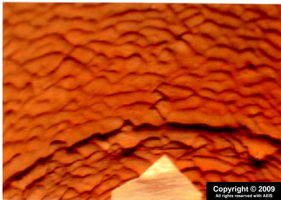
Figure 2: Internal Surface of the Spool Piece and the Suspected Crack
