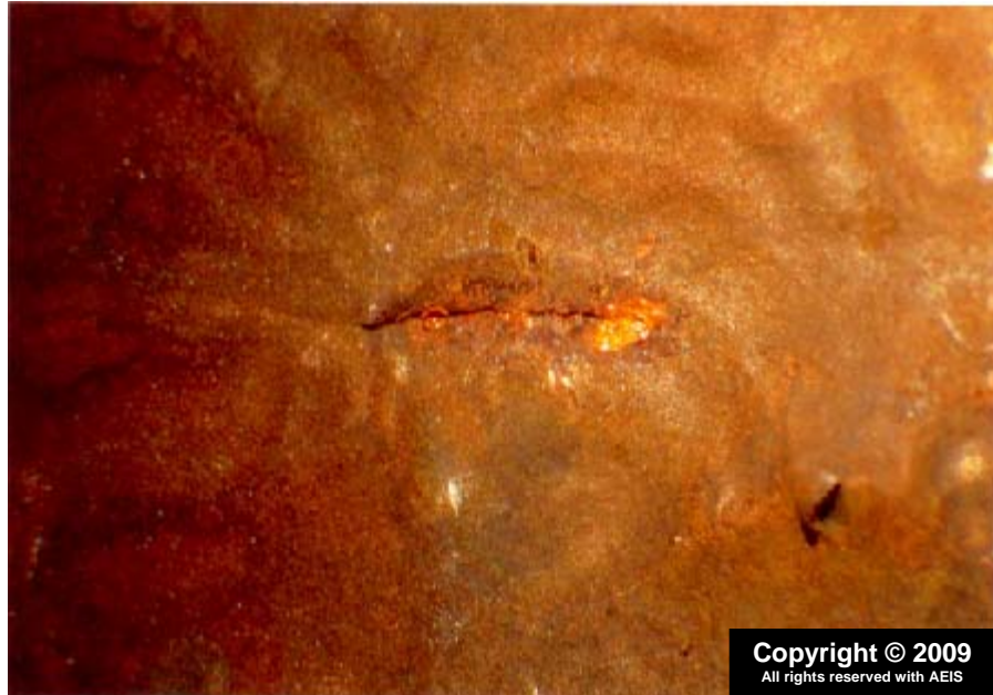
Figure 4: Another Crack Lip on the Inside Surface.
